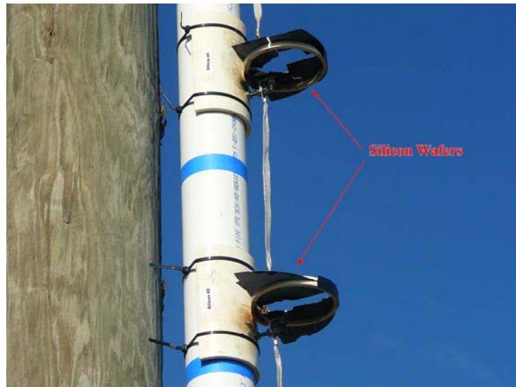
Figure 6. Lightning-damaged Silicon Wafers
